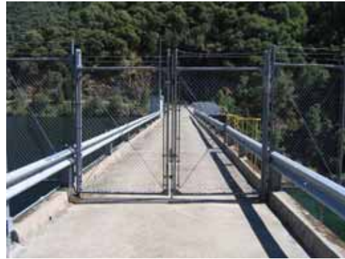
RADRAAP01 – Ralston Afterbay Dam Road and Afterbay Access Point at Road Mile 0.021
