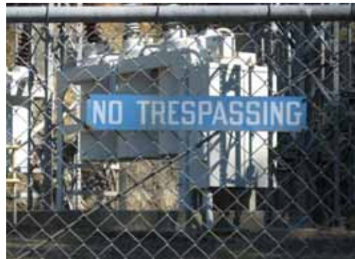
MFPUSR01B – Middle Fork Powerhouse Upper Switchyard Road (no Road Mile data collected)
