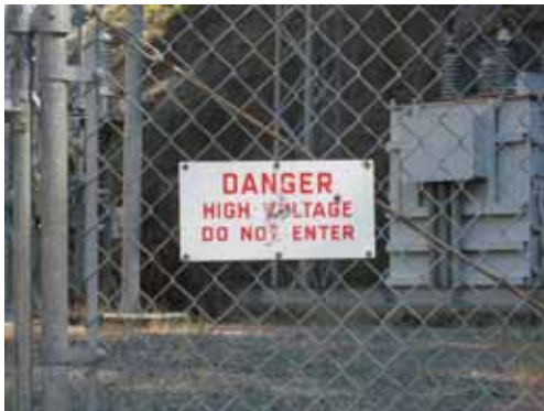
MFPUSR01A – Middle Fork Powerhouse Upper Switchyard Road (no Road Mile data collected)
