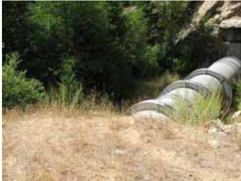
NFLCCRSNRPA07 – North Fork Long Canyon Crossing Removable Section North Road and Parking Area at Road Mile 0.145
