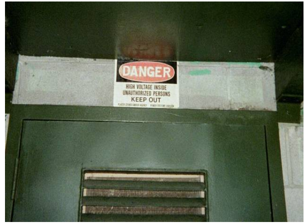
Photo 4. Sign is located on the Hell Hole Powerhouse on the wall above the front entrance.
