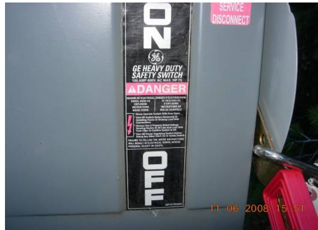
Photo 20. Sign is located on the electrical box on a power pole near Middle Fork Powerhouse Butterfly Valve House.
