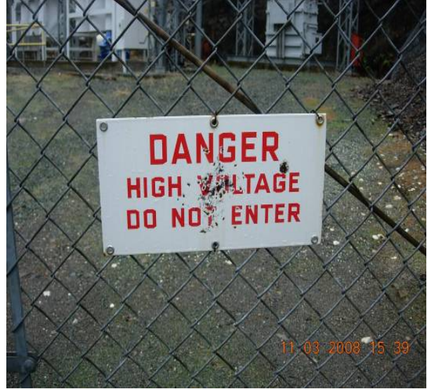
Photo 22. Sign is located at the main access gate and fence to the Middle Fork Powerhouse Upper Switchyard.
