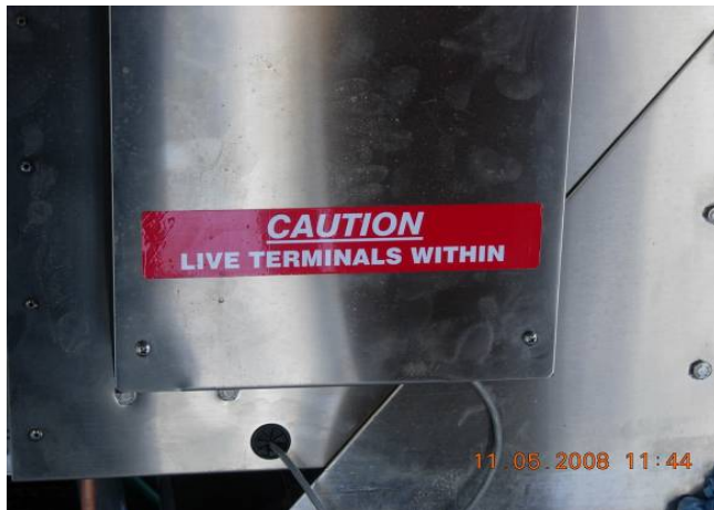
Photo 19. Sign is located on the faceplate of generator at Duncan Creek – Middle Fork Tunnel controls platform.
