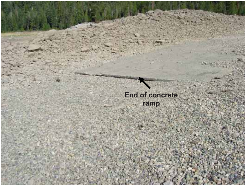
Photo H-8. McGuire Boat Ramp on September 24, 2008 (WSE = 5,198 ft). Note that end of concrete ramp is at 5,200 feet.
