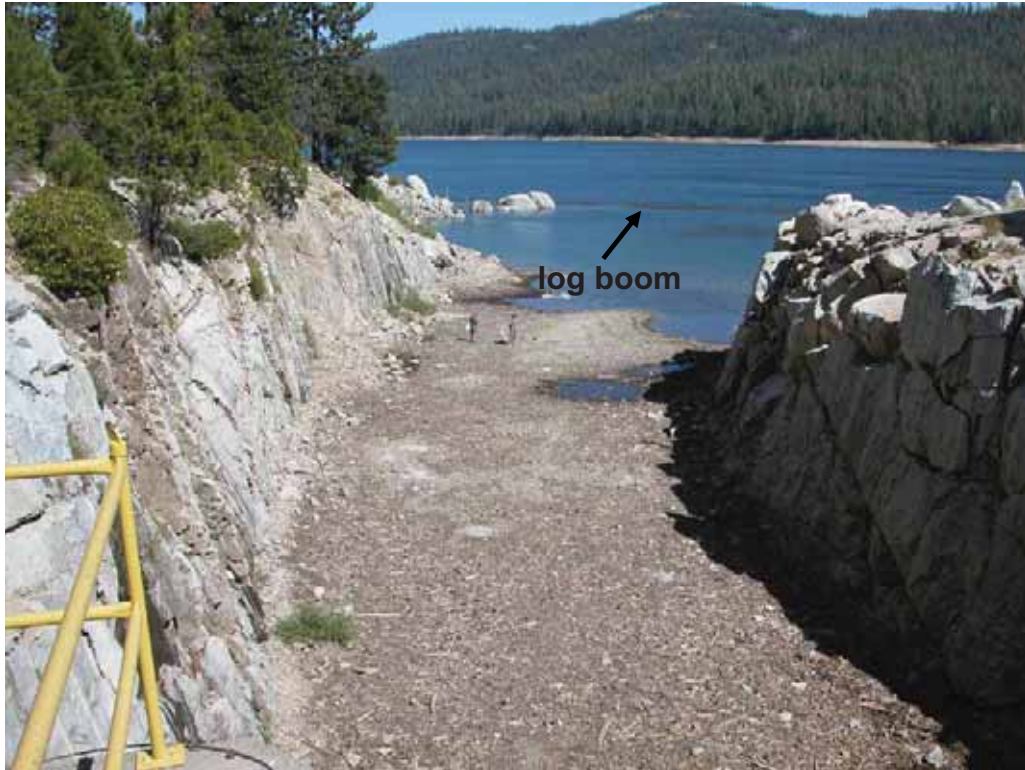
Photo J-1. View of log boom near spillway at French Meadows Reservoir.
