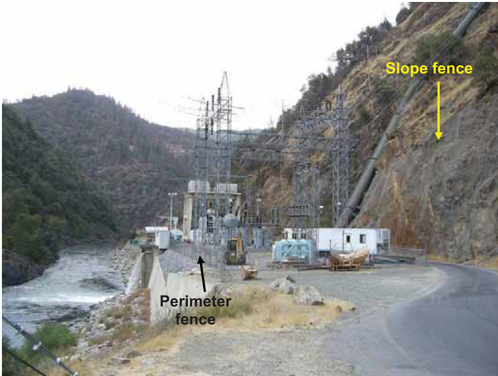
Photo M-2. View of public safety fence (perimeter fence) surrounding Ralston Powerhouse. Also note slope fence along road way. The slope fence is prevents rocks from falling on to the roadway.
