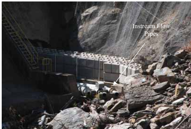
Middle Fork Interbay Dam - Instream Flow Pipes
