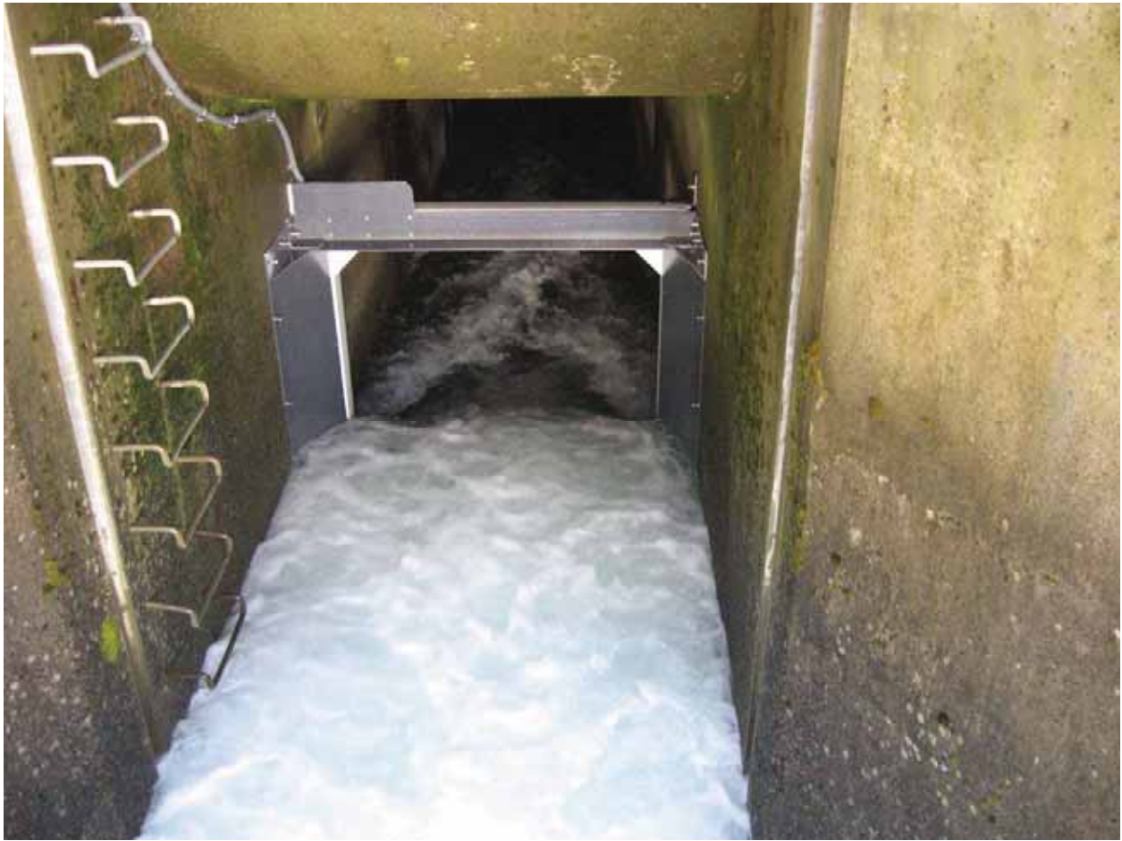
Photograph E-2. Duncan Creek Antenna in Diversion Tunnel.
