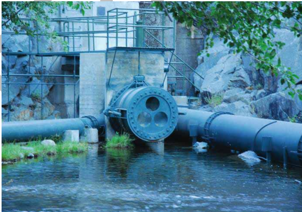
Dam Low Level Discharge Ring Jet Valve
