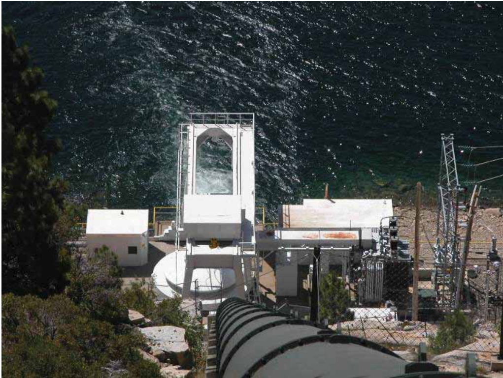
French Meadows Powerhouse
