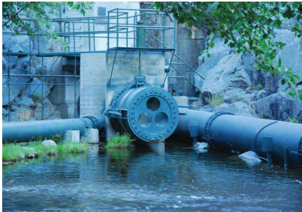
Dam Low Level Discharge Ring Jet Valve
