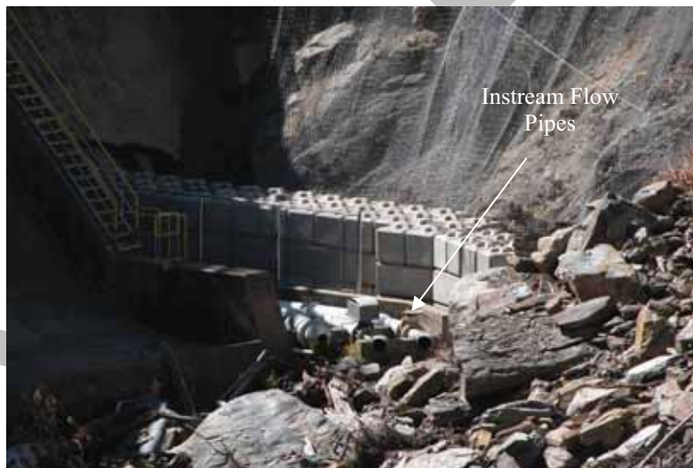
Middle Fork Interbay Dam - Instream Flow Pipes
