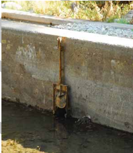
North Fork Long Canyon Diversion - Instream Flow Pipe
