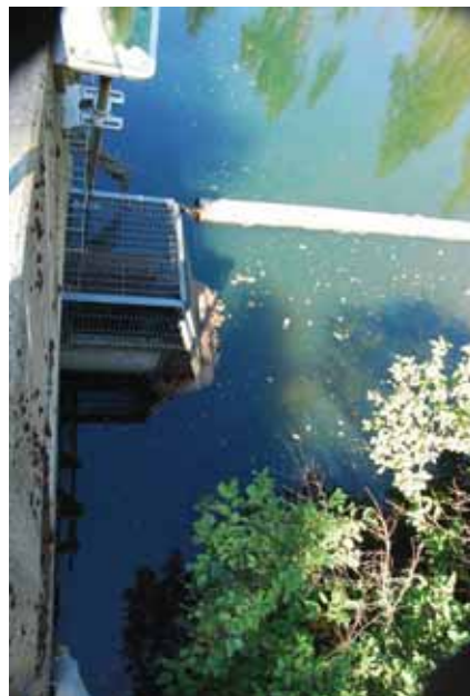
Inlet to Instream Flow Pipe
